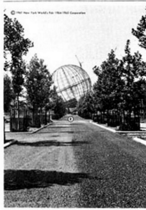
The Unisphere®, with all structural steel in place, as seen from the Avenue of the Americas last week.
