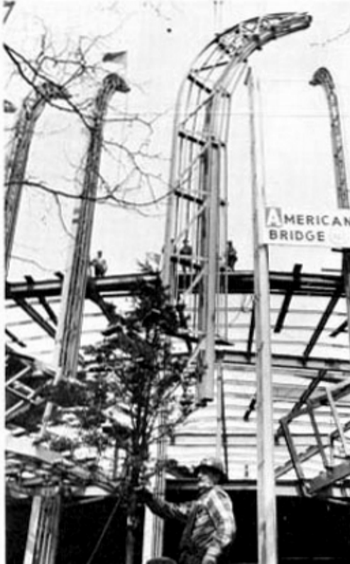
A two-ton top section of a 100-foot high pylon as it was swung into place over the Rotunda entrance of Ford Motor Company's Fair Pavilion to mark completion of structural steel erection on the massive building. Workers of U.S. Steel's American Bridge Division later went aloft to plant a six-foot fir tree, appropriately decorated with miniature automobiles, and a World's Fair flag. Shown is steel worker, Jay Feltham holding the traditional "topping out" tree.
